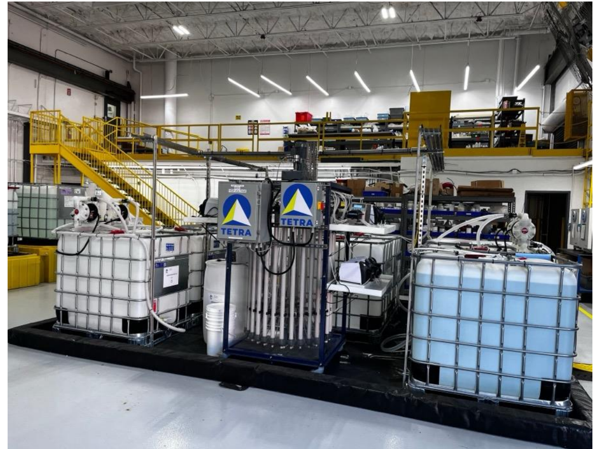
Iodide Extraction Pilot Unit TETRA Innovation Group
