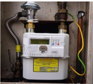
Water & Gas Meters
